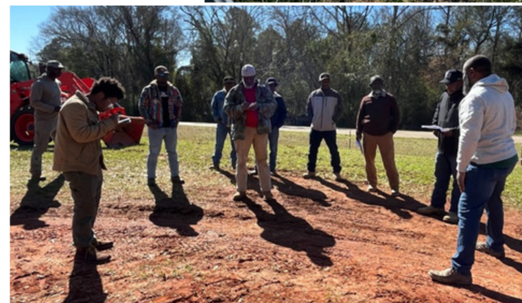
Below: TUCCA Rep. Darrel McGuire (far right) leads an on-site installation demonstration for farmers. Dallas County
