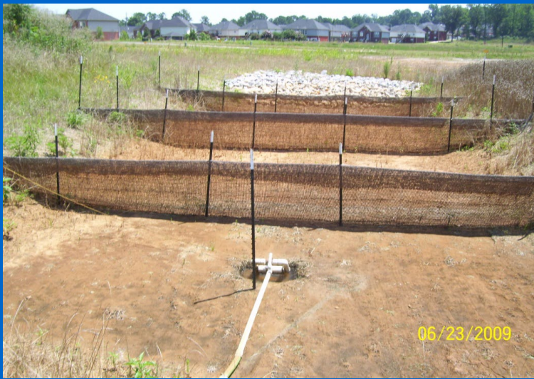
Bessemer – 1 st Sed Basin with baffles, skimmer, flocculant
