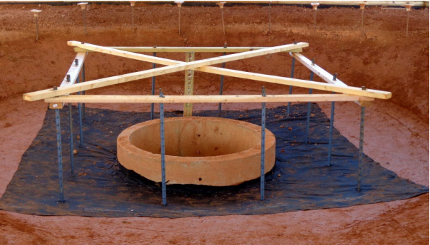
Figure IP-1 Silt Fence Inlet Protection installation showing geotextile underlayment, steel T-posts, 2 x 4 bracing, and dewatering device.
