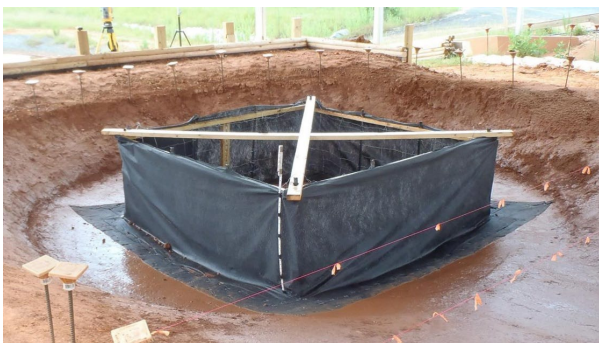
Figure IP-2 Silt Fence Inlet Protection installation showing silt fence, geotextile underlayment, steel T-posts, 2 x 4 bracing, and dewatering device.
