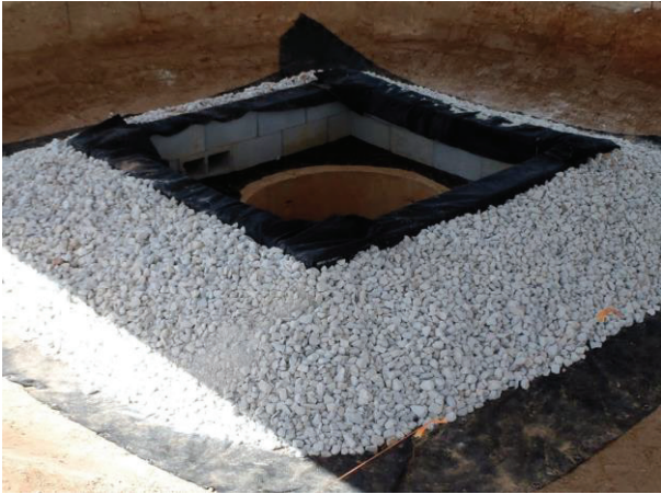
Figure IP-3 Block and Gravel Inlet Protection installation showing geotextile underlayment, gravel, and dewatering device. (Photo courtesy of AU-ESCTF)
