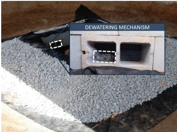
Figure IP-4 Block and Gravel Inlet Protection installation showing dewatering device. (Photo courtesy of AU-ESCTF)
